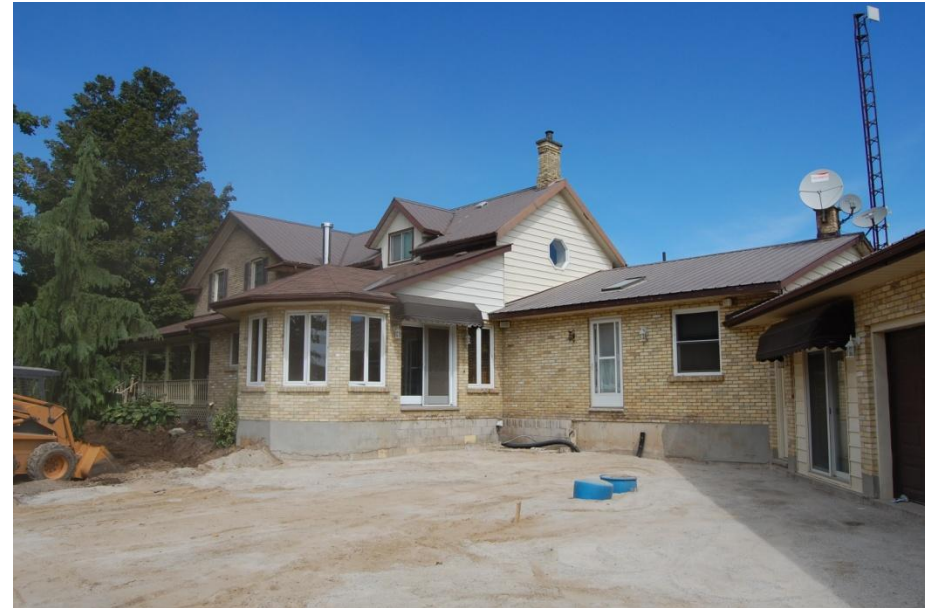
Figure 9 – Tail and rear additions. (Photo: RHC, Aug 2012)
